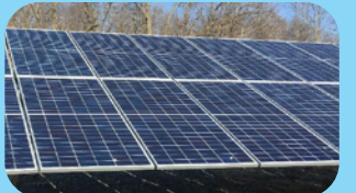
Two solar arrays were installed on city property.
