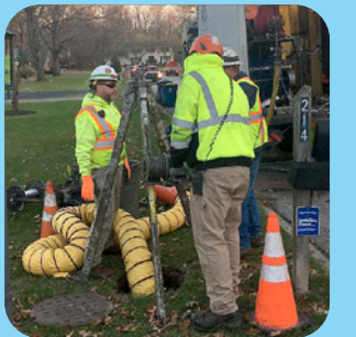
Adding lining to existing pipes to extend the life of the sanitary sewer pipes.
