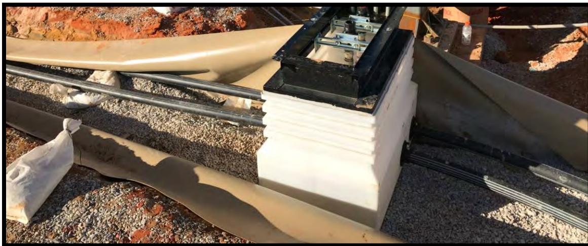
2 – Example image of liner being installed around and under double wall piping, providing tertiary containment for the fuel storage and distribution system.
