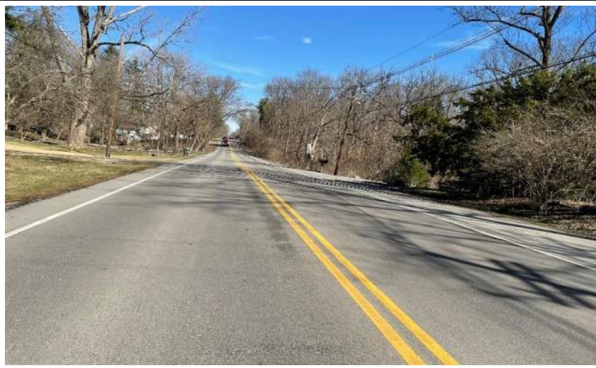
Photo 1. Looking north up Westfield Blvd., approximately 0.16 mile north of the 106 th Street and Westfield Blvd. intersection.
