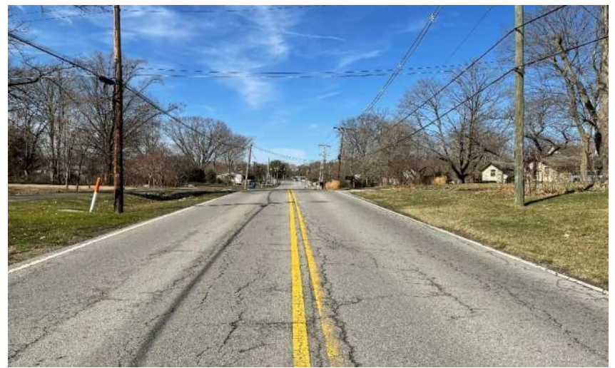
Photo 20. Looking west down E. 106 th Street, approximately 0.14 mile east of the intersection.
